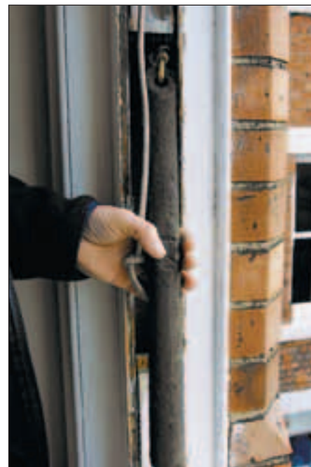
Sash windows: UPVC detract from the character of older houses
